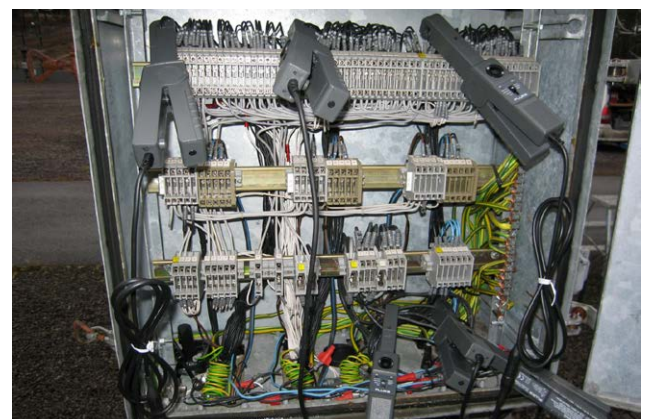
Figure 3 Control cabinet with current clamps
