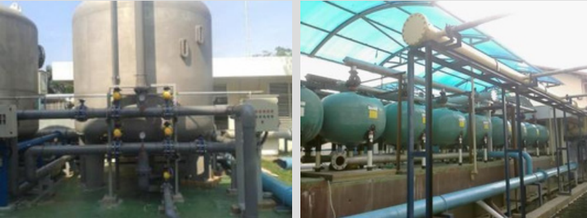
DRINKING WATER Cap 200 L/s – Jakarta
