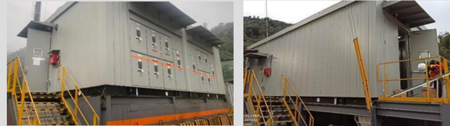
Electrical Housing Mining Papua
