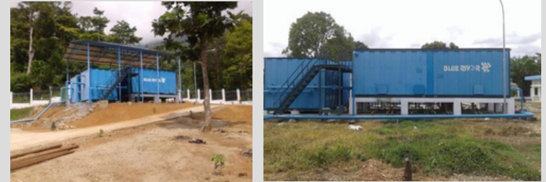
WATER TREATMENT PLANT, Cap 2 X 10 Liter/detik - Aceh
