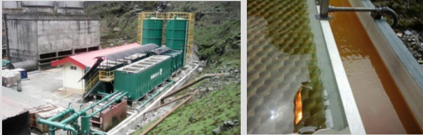
WATER TREATMENT PLANT 2X20 Lps Papua
