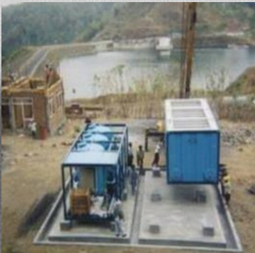
Water Treatment Sumatera
