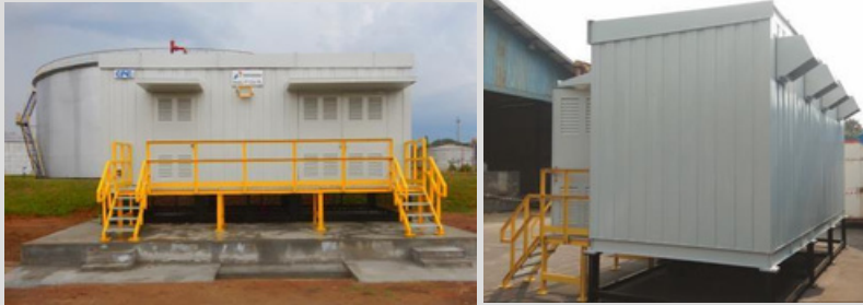
Container SS – Diesel Power Plant | PLTD JAKABARING
