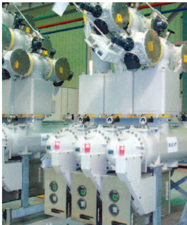
High Voltage Switch Gear in AREVA Suzhou (China)
